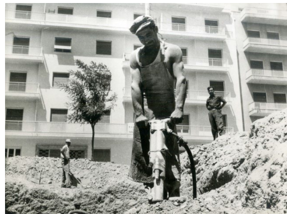
Fig.1: Builders working for the construction of polykatoikia buildings, Athens, ca. 1950s. (Source: Megaloeconomou Archives, Benaki Museum).
